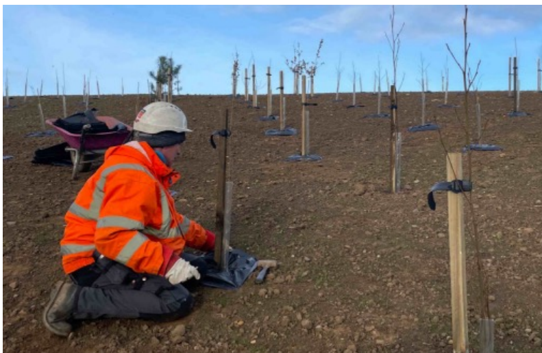
Example of revegetation underway at converter station site (Sofia and Dogger Bank C)
