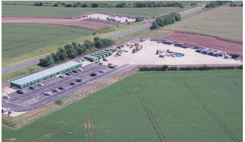
Example of a construction compound for onshore cable installation works (Sofia and Dogger Bank C Offshore Wind Farms)
